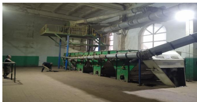
Figure 1. View of the existing aspiration system of the UHK aggregate at the "Angor" cotton processing plant,
